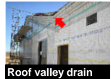
Roof valley drain
